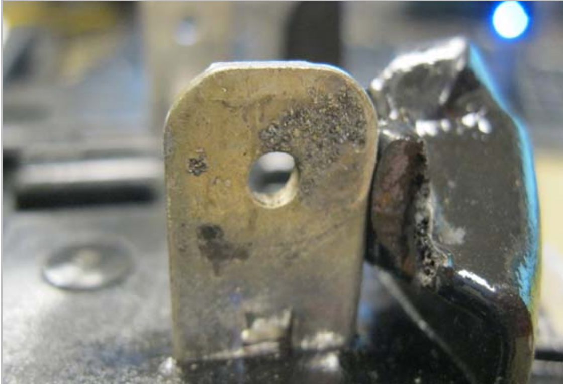
Figure 1. Pitting and Discoloration of a Hot Socket Meter Stab Returned from the Field
